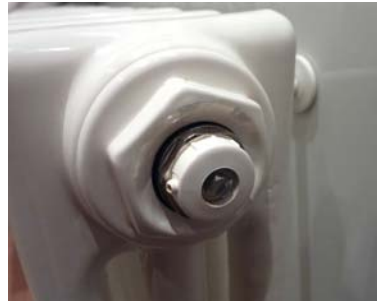
Radiator showing bleed valve
